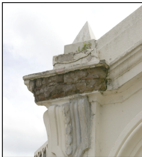
Damage to the Bath House (gazebo)
